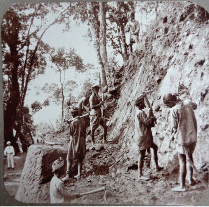
Figure 1. A New Mission Road is Cut into the Hill above a Government Road, Serkawn, 1913
