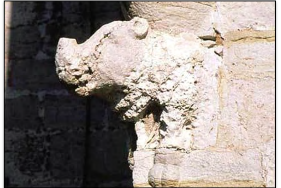
The rhino gargoyles can still be seen on the Belém Tower, but unfortunately are very badly weathered.
