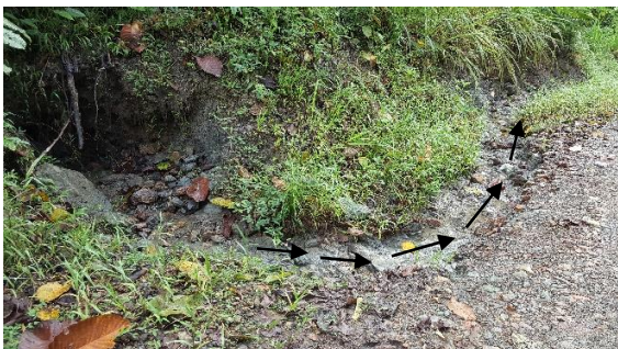
Plate 3. The erosions and redirection of water flow (arrow)
