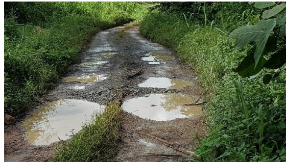
Plate 1. Puddles seen on the road between RQF and RIF, in Tabin
