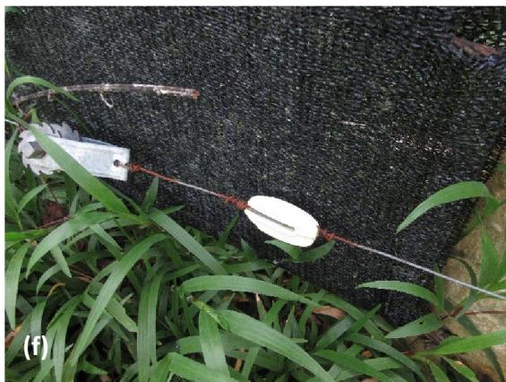
Plate 24 (d). Rusty broken substandard fence wires, (e and f) substandard wires used for insulators
