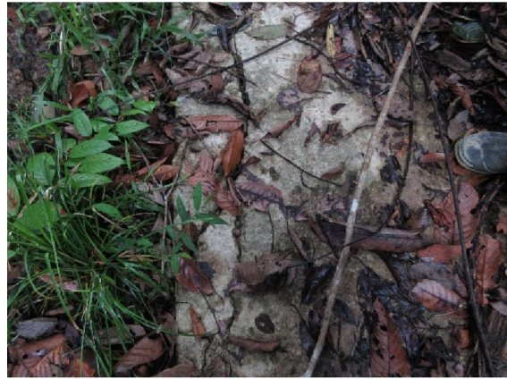
Plate 30. Cracks were seen at the pavement of the culvert
