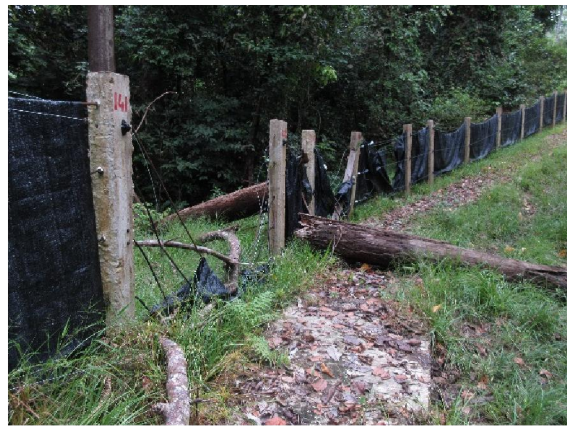
Plate 24. The broken fence line due to previous tree fall
