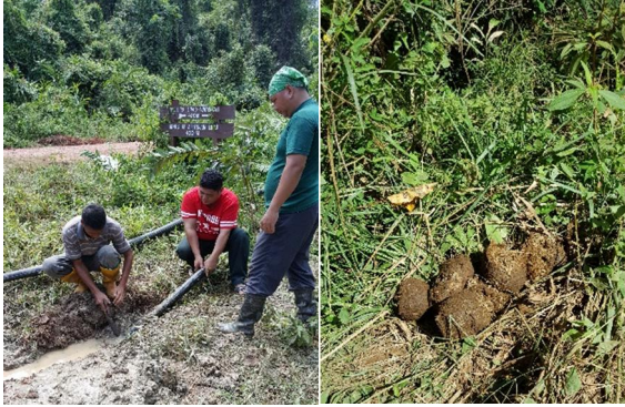
Plate 1. The damaged pipelines (a) and elephant dung piles (b)
