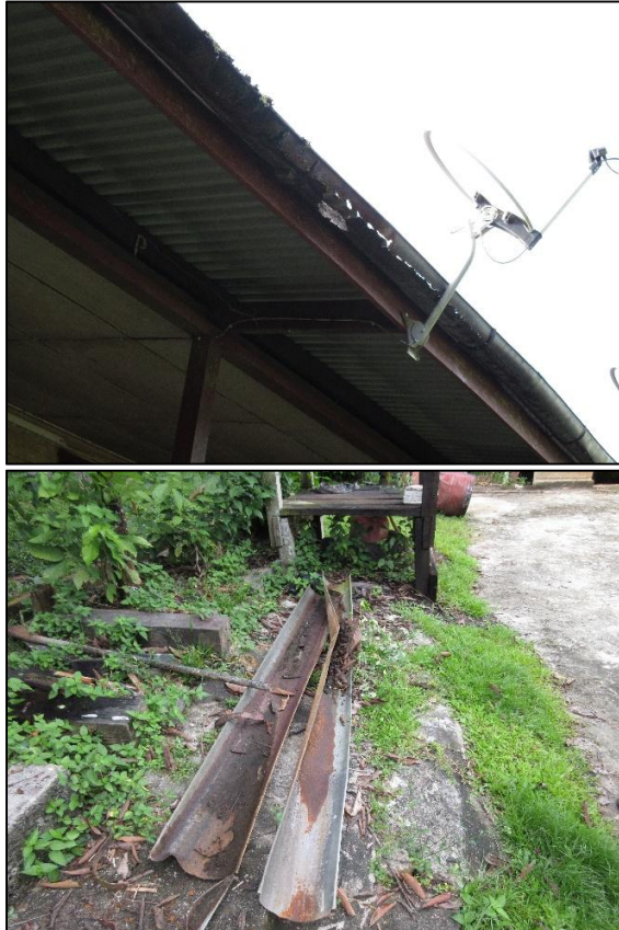
Plate 19. The leak holes on the gutters (above) and the rusty gutters (below)
