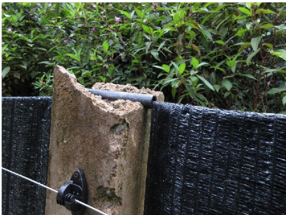
Plate 23. One of the broken concrete post
