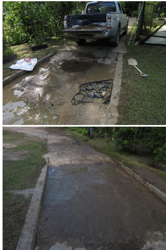
Plate 20. The damaged tyre bath (above) and (below) after it was repaired
