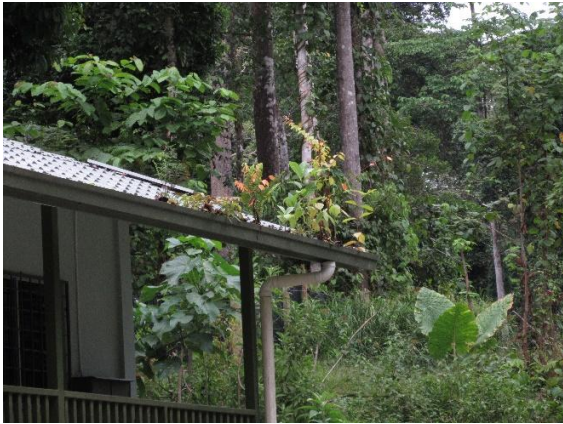
Plate 33. The Laran tree ( N. cadamba ) and ferns growing on the roof of the staff quarters
