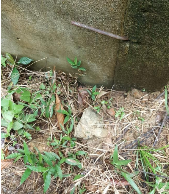
Plate 18. The concrete based next to the wall are sharp and difficult to be removed. Need to be hacked. Note the rusty metal piece from the wall which was only visible after weeding
