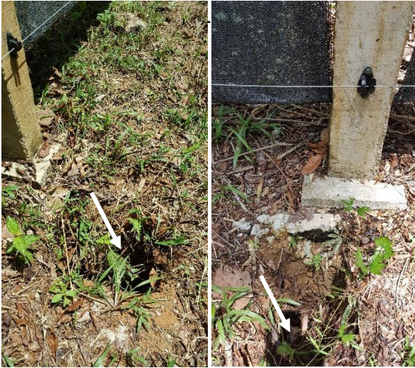
Plate 14. The uncovered one – meter deep holes next to the concrete post. Danger to the keepers and rhinos
