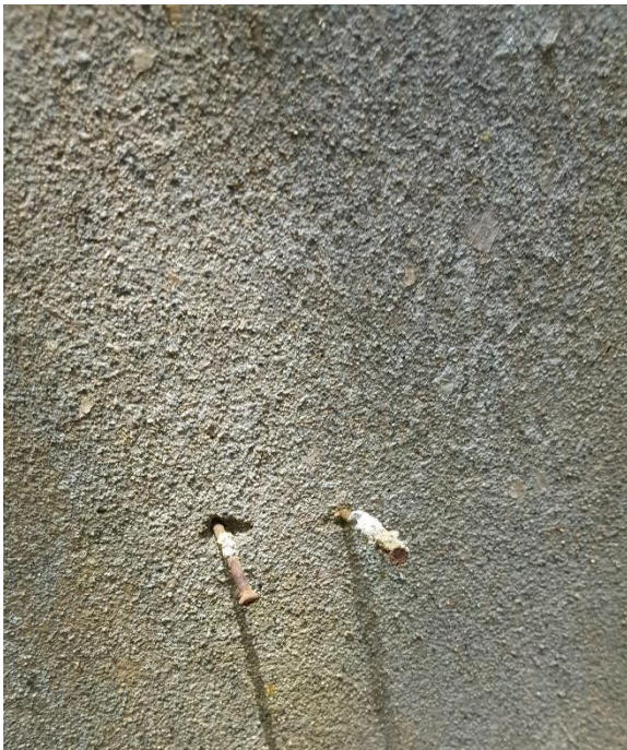
Plate 19. The nails jutting out from the concrete wall
