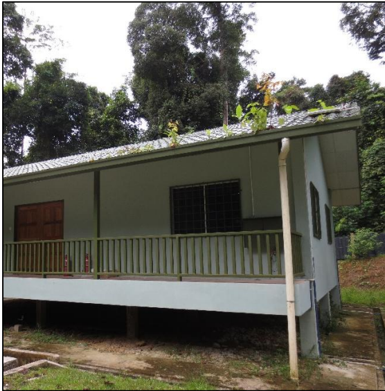
Plate 27k. The roofing gutter is filled with growing Kelawit ( Uncaria spp ) and Laran ( Neolarmakia cadamba ) seedlings. These should be cleared by the contractors prior to it being handed over to Sabah Wildlife Department.
