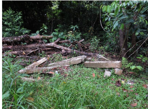
Plate 27j. The left over from the contractual work could still be found inside and outside the paddocks. Some are potentially very dangerous to the rhinos. There should not be any of the construction materials left in or outside the BRS facility as it is within the Wildlife Reserve.
