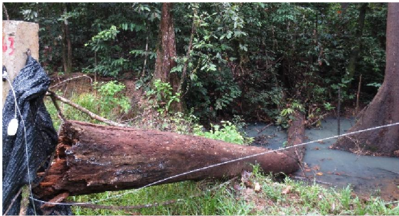
Plate 27f. The fallen tree on the electric fence occurred about six months ago and never cleared. The sagging on the fence will become permanent if this is not cleared.
