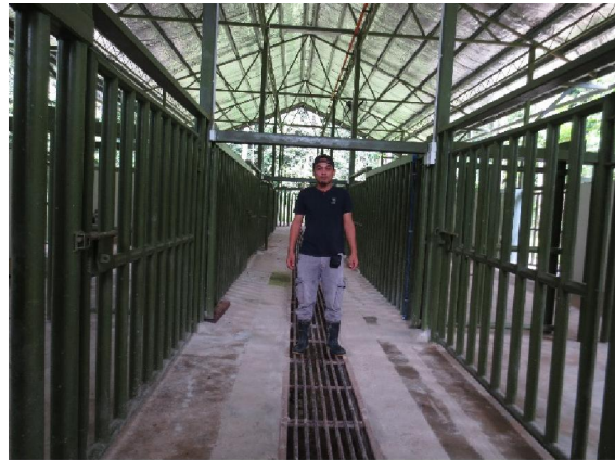
Plate 27i. The 3% slope on the flooring of the night stall has not been rectified. This will pose a problem in managing the health and hygiene of the rhinos in captivity.
