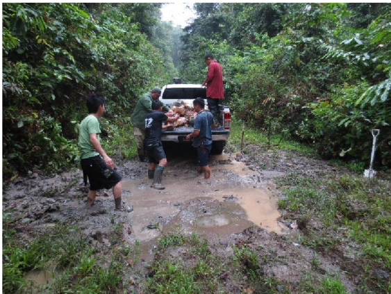
Plate 1. Collecting the cement blocks (a) and (b) filling up the damaged road
