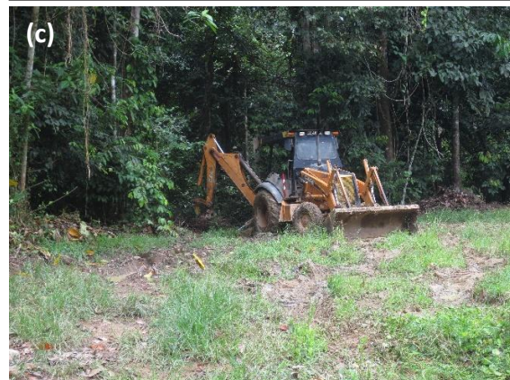
Plate 16. The KL – Kepong bulldozer making drains (a), repairing a bridge (b) and clearing the composting site (c)
