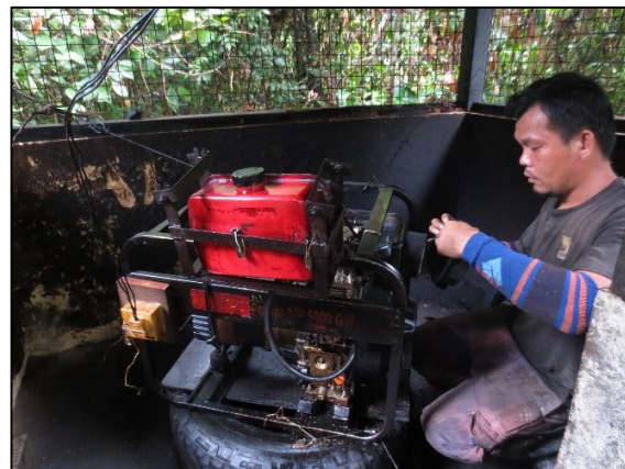
Plate 21. James Sandiyang repairing the generators in RQF (a) and RIF (b)
