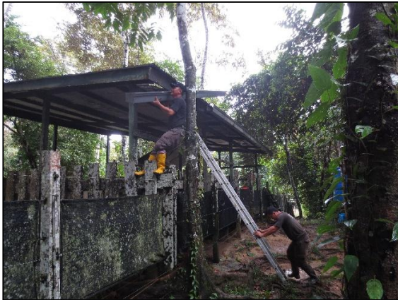
Plate 22. Joseph removing the gutter to clean while Alvin (above) uses a rake to remove leaves from another end
