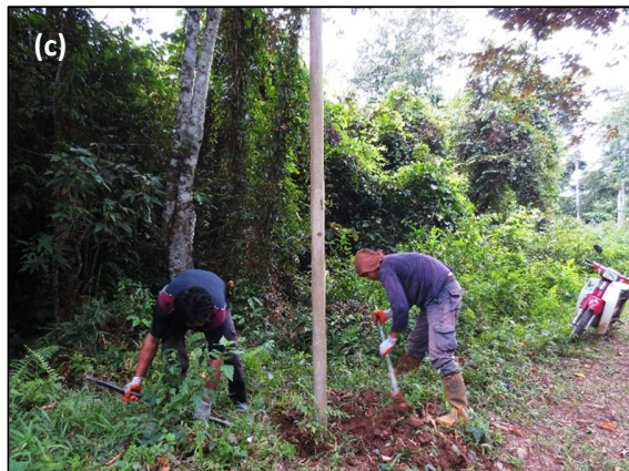
Plate 19. Removing the electric wires from the post (a), rolling the wires (b) and (c) removing the GI post
