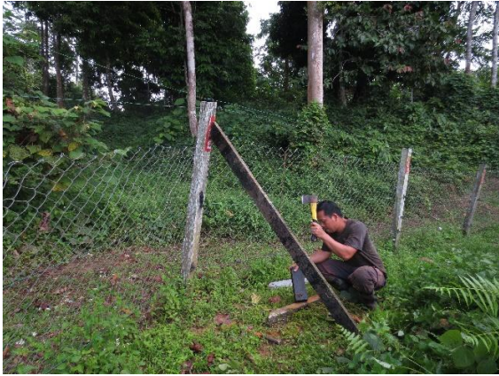
Plate14. James installing a brace against a tilting post in the Rhino Food Plantation
