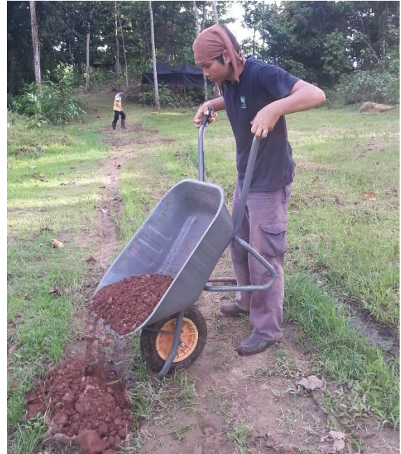
Plate 10. BORA staff using a wheel barrow to fill up a wet patch.
