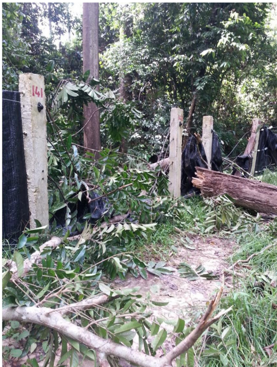
Plate 26. Tree fell onto the fence
