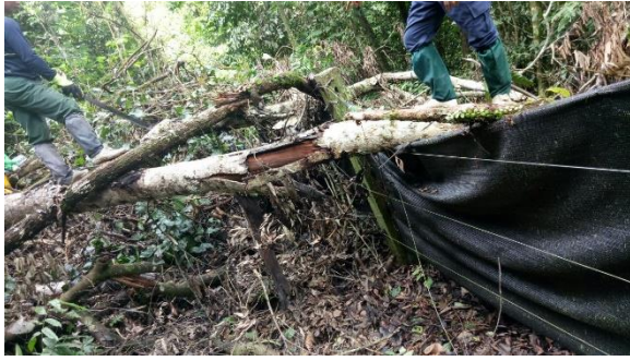
Plate 16. Tree fell that damaged the fence and being repaired by BORA staff
