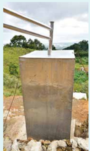
Condenser unit for stream vent
