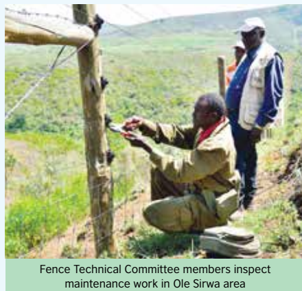
A fence attendant carries out maintenance work on the fence in Ndabibi area
