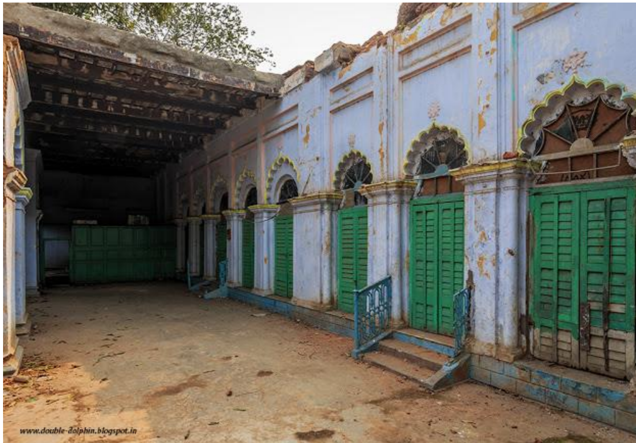
Bait-un-Nijat's collapsed roof
