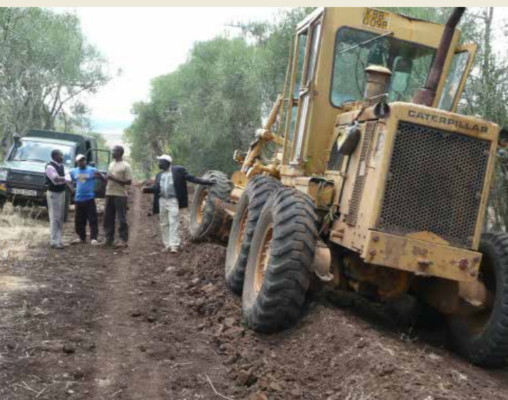
One of the ways in which Lewa promotes infrastructure development in the neighbouring communities is through the grading and repair of community roads. © Natalie Solveland
