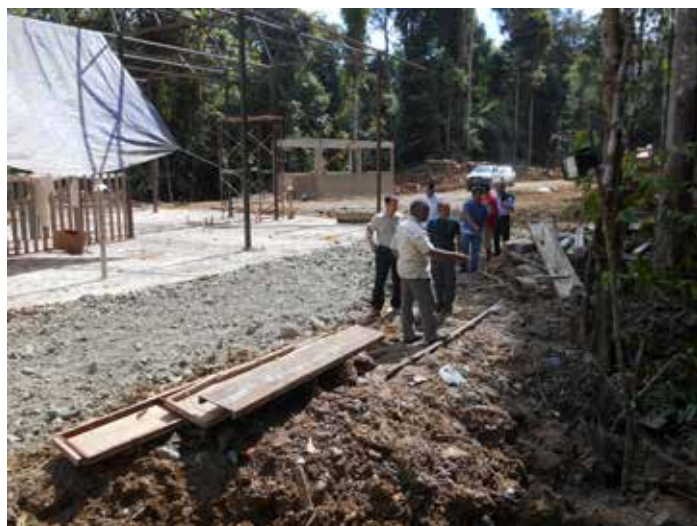
Ministry of Natural Resources & Environment and Department of Wildlife & National Parks Malaysia officials visiting the BRS facility under construction in Tabin Wildlife Reserve, August 2014.
