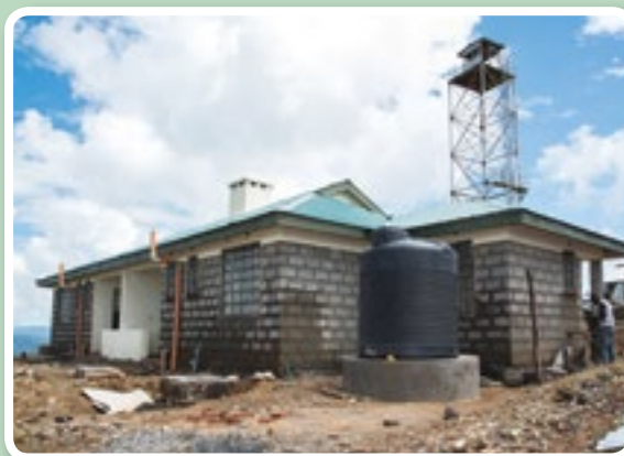
View of the Fire Watch Tower fence energizer house
