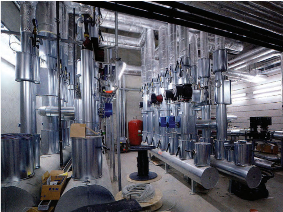
Utilities room where Gondwanaland is connected to the district heating network.
