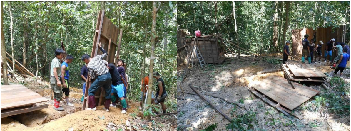
Construction of the boma, 11 March, collaboration involving BORA, Wildlife Rescue Unit, Sabah Foundation staff and others, (left) placement of sections of hardwood fence into the perimeter trench, (right) Iman inside the crate on the left with fence construction ongoing to the right.
