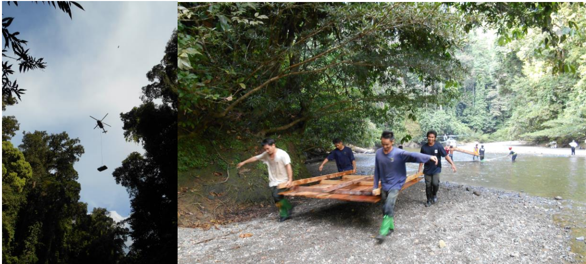
(left) view of helicopter bringing a batch of materials to the drop site, (right) moving sections of boma from the drop site to the temporary storage site, 23 July (staff Marikus Suyat, Tinrus Tindok, Suzali Jaya and Zuraimi Rahman)
