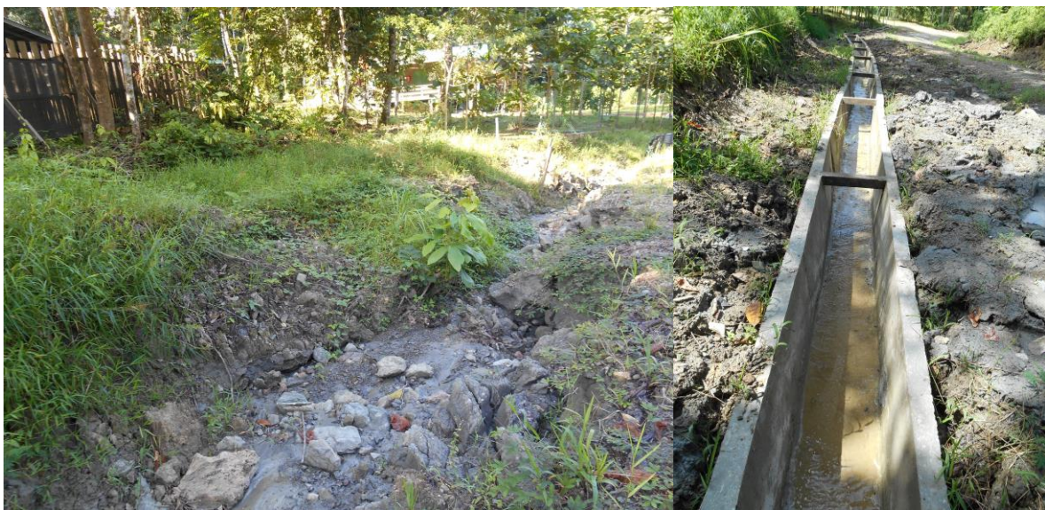
Road next to the interim rhino facilities at Tabin, (left) a drain dug in 2012 eroded to this by July 2013, (right) the concrete roadside drain completed in early October
