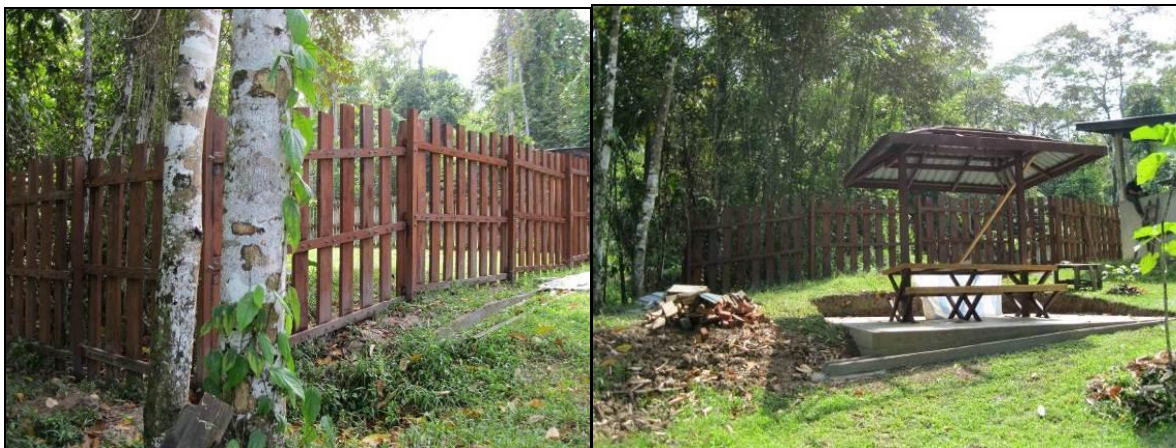
(left) external view of the rhino breeding yard fence at the rhino interim facilities, completed at end of June, (right) one of two gazebos completed in June at the rhino interim facilities
