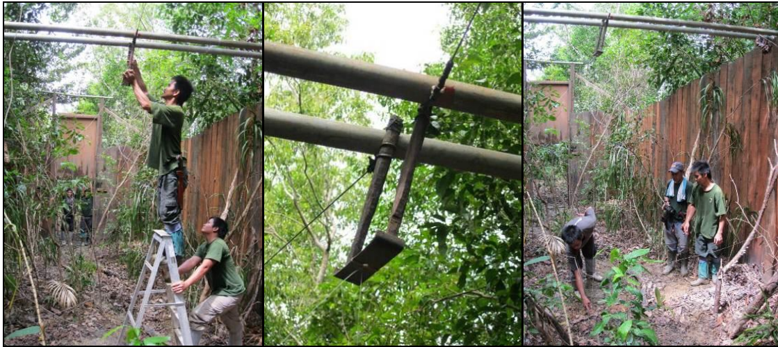
(left) the inside end of each cable is tied to an ironwood peg, (middle) close-up view of the final trigger design, with ironwood pegs held in place by a combination of galvanised iron cross pipes above and, below, a steel plate with a flange at each end, (right) when a large animal enters the trap, it will push an arrangement of barely-visible, fine plastic-coated wire, that pulls the steel plate downwards and simultaneously releases the ironwood pegs, cables and doors within 1 second.
