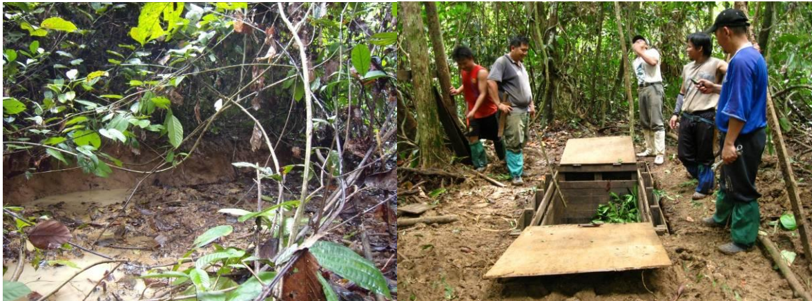
(Left) A mud wallow used by Puntung at Malambabula, (right) new trap for Puntung (trap 4, near to a rhino wallow), in process of construction, 20-22 January (© Herman Stawin).
