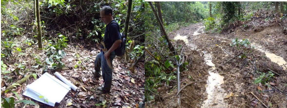
(Left) BORA field manager / veterinarian views the proposed permanent BRS breeding facilities site. (Right) Initial construction work on the 1.2 km access road to the BRS breeding facilities (25 November 2010, note effects of rain).
