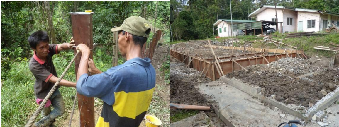
(Left) Re-construction of Tam's forest paddock to become two adjacent paddocks. (Right) Commencement of re-construction of the old kitchens/store at Tabin to become staff accommodation (18 February).
