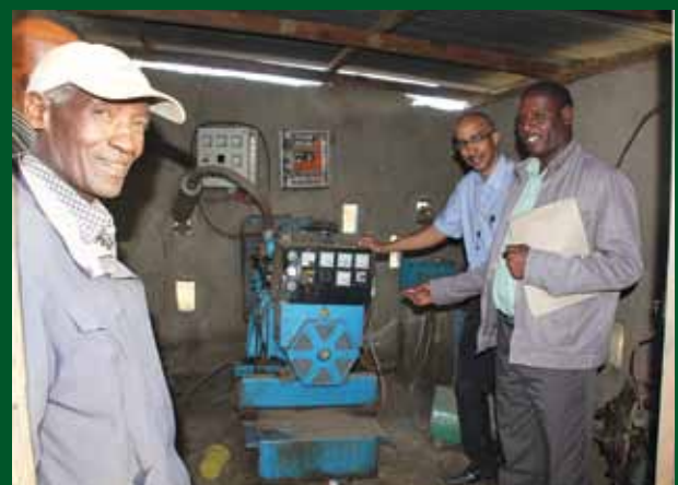
Inspecting generator unit at Shamba Boy borehole
