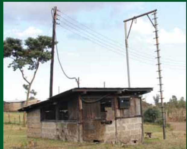
Ndibithi borehole pump house
