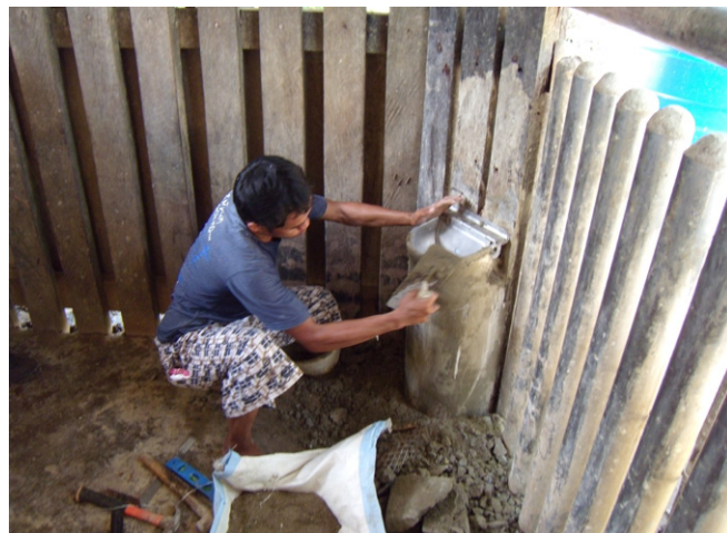
Automatic water dispensers were fitted into the interim rhino paddocks at Tabin in September 2010, to provide constant clean drinking water for the rhinos.
