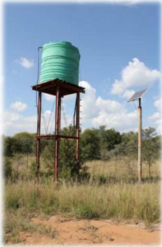
Borehole with solar panel and tank
