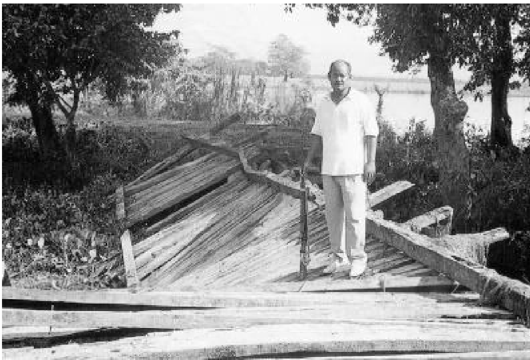
A damaged bridge with Mr D. Boro, the Range Officer in central Kaziranga.
