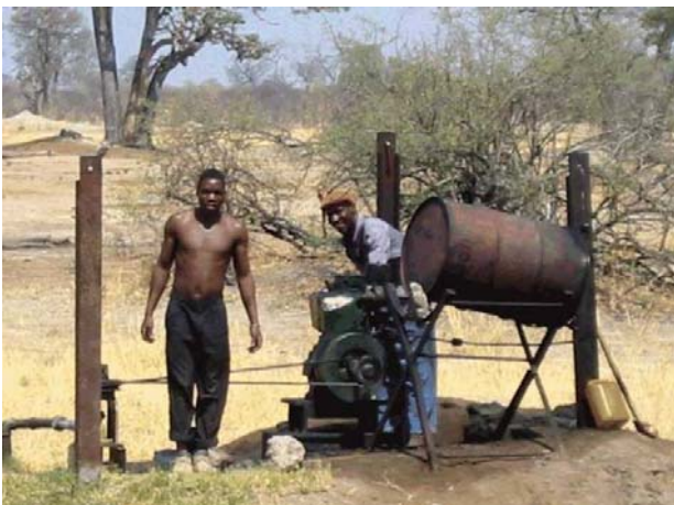
Pump attendants in need of spares and diesel.
